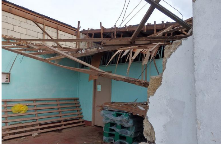
Damaged roof at Bantayan District Hospital
